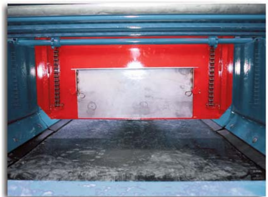
GUILLOTINE SHUTTER IN REST POSITION
